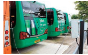
With an ABB Terra 51 fast-charger at the main car park, Travel De Courcey can re-charge its Versa EVs to full capacity in less than two hours
